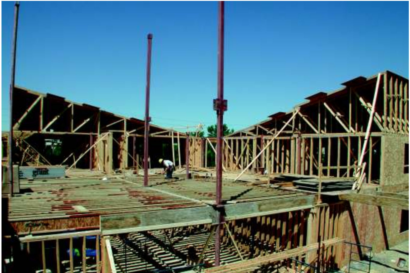
PHOTO 3: Numerous types of light wood-frame building systems are available to maximize fire safety and minimize sound transmission.
